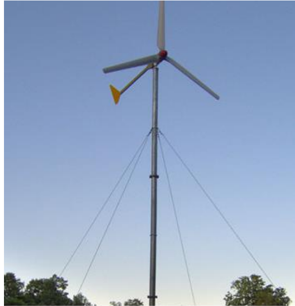
Guyed Pole Tower
